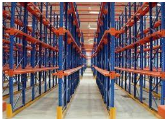
Gambar 2.4 Drive In Racking System
